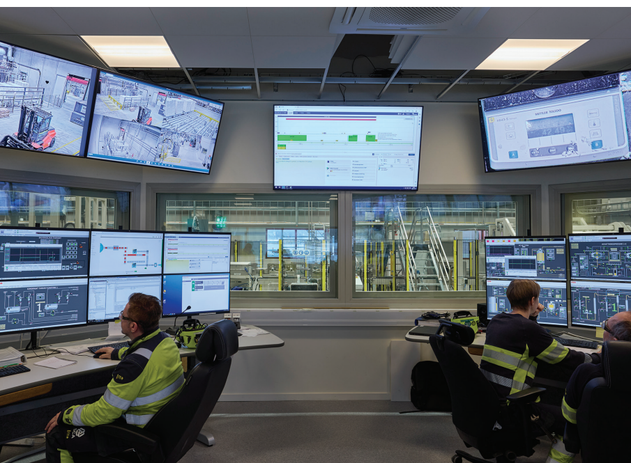
Figure 11: Inside control room.
